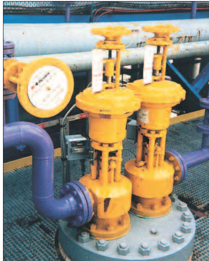
Liquefied gas storage valves Model 2200.
